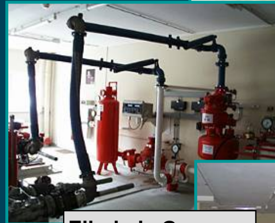
Ellerbek, Germany facility
